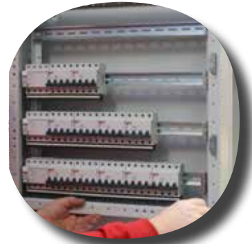
Cables and front frame are fitted.
