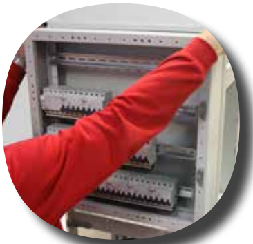
Flanges are fitted in top and bottom.
